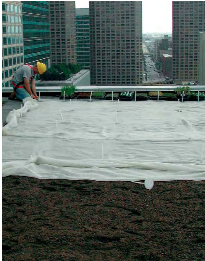
■ A certified green roof professional ensures all green roof components are installed properly. Some manufacturers also offer training programs for installation contractors about the proper use of materials. Photo courtesy of American Hydrotech.
