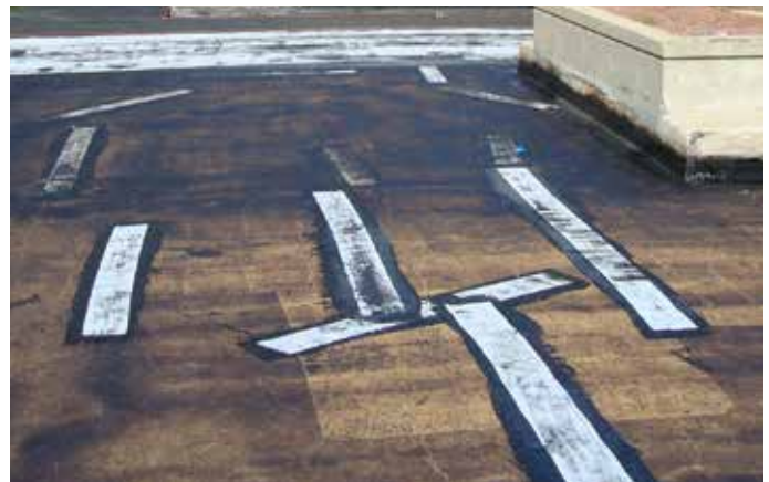
Shrinkage cracks > 1/16" and < 1/4"
